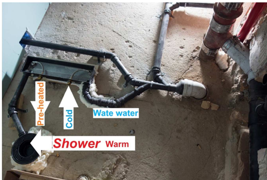
FIGURE 3-8: INSTALLATION OF DRAIN-WATER-HEAT-RECOVERY HEAT-EXCHANGER IN THE BATHROOM OF BEST NBR. 3
